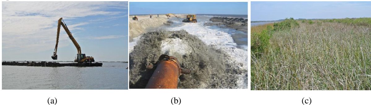
Figure 1: The Sabine Refuge Marsh Creation Project, (a) construction of the dike, (b) dredged riverine sediments pumped to the open water area, (c) newly created marshland
