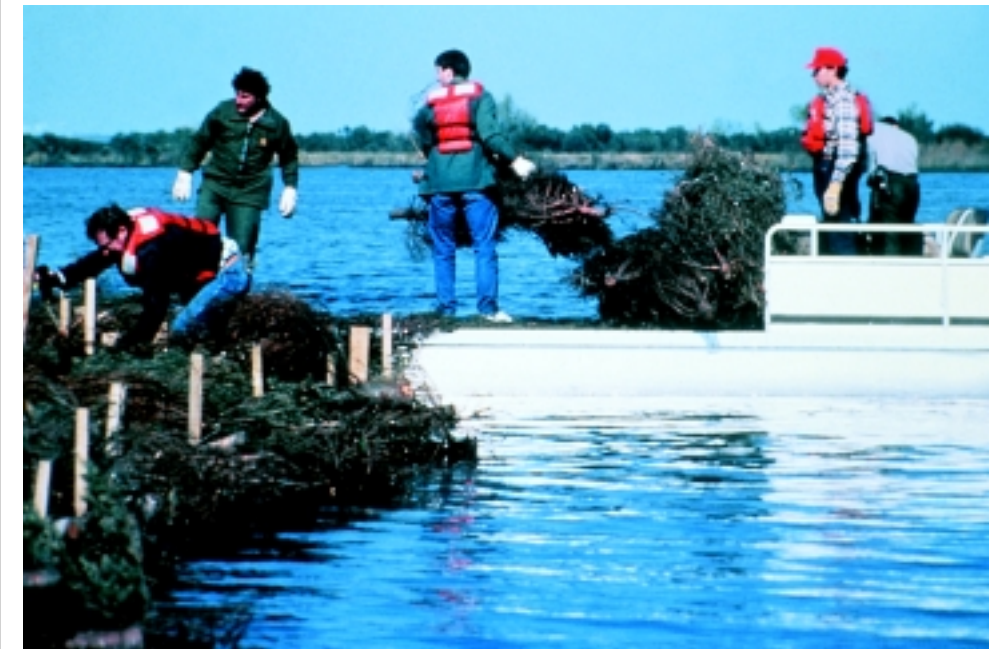
Building a Christmas tree fence. Photo courtesy of Coastal Restoration Division, DNR.
