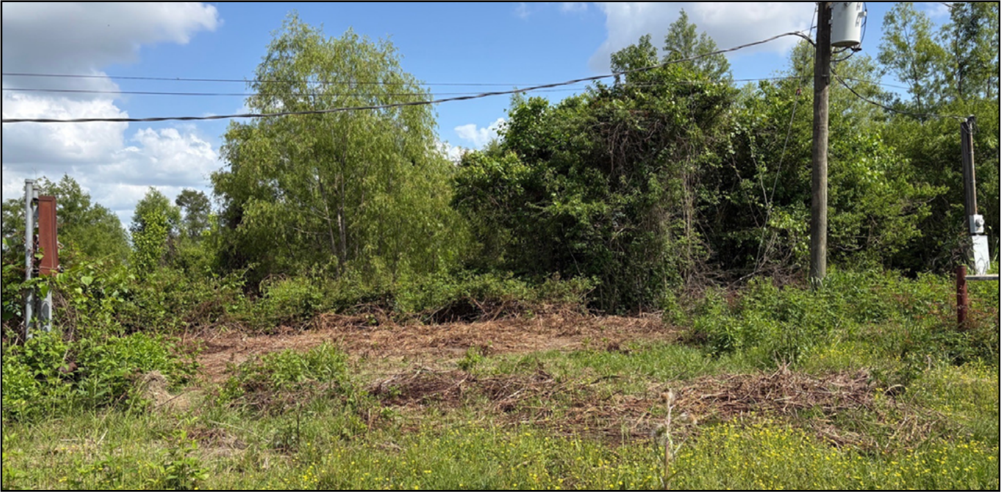
The clearing by the marine research building that RNR 4022 students made by clipping and removing thick, overgrown vegetation to access the power line to restore power.
